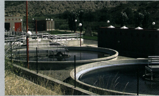
Treatment Plant in Flix
